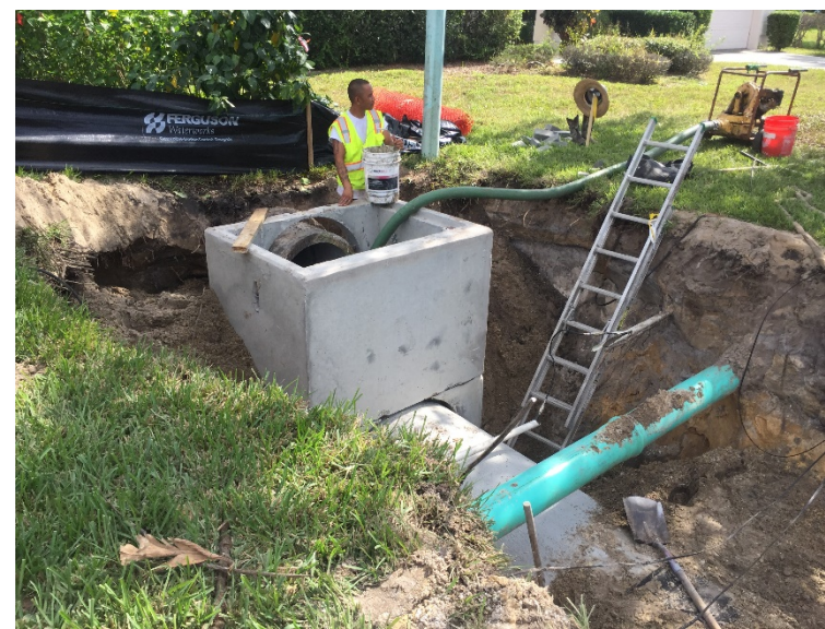
Ditch bottom inlet (Riverside Drive – Tarpon Springs)
