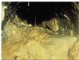
Grease buildup on the interior of sewer line.
