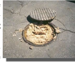
Excessive grease from overflowing manhole
