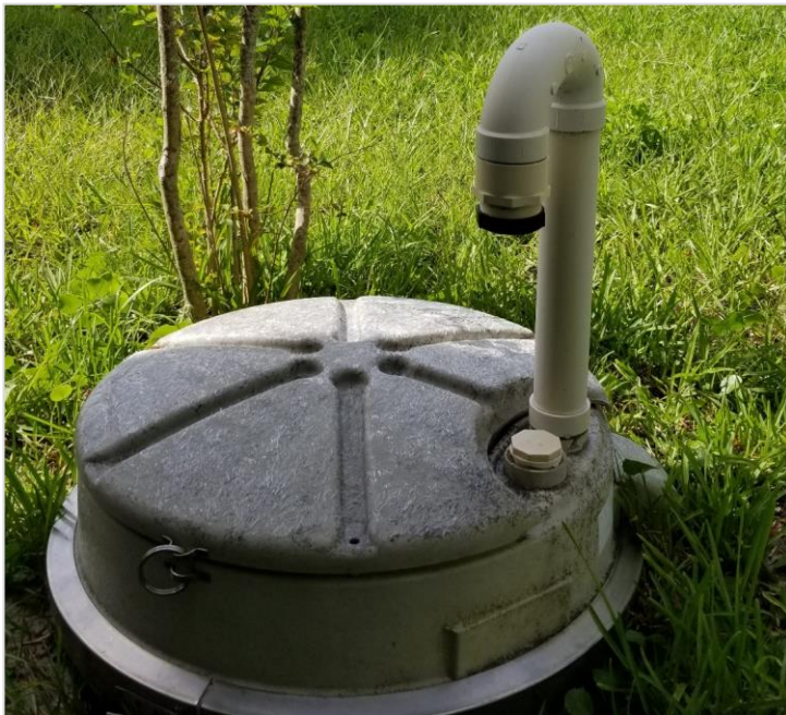
Figure 3 Grinder Pump Station Flood Proof Cover and Vent
